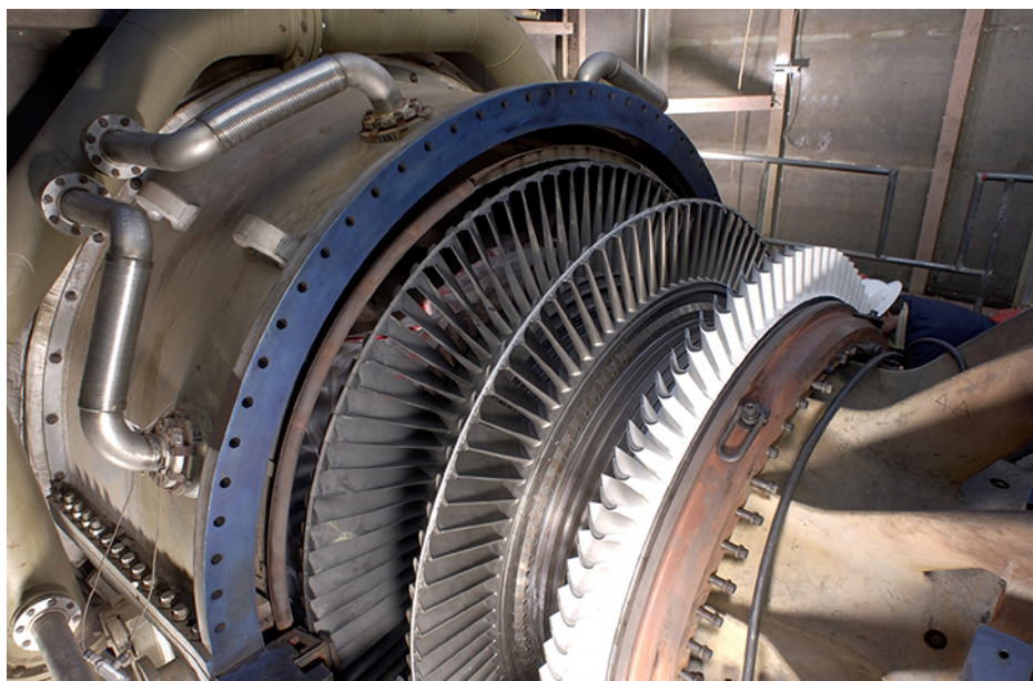
Figure 13.31 Steam turbine/generator. The steam produced by burning coal impacts the turbine blades, turning the shaft, which is connected to the generator.
