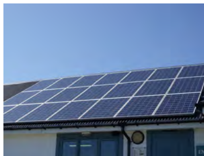
Figure 12.1: The use of solar cells to supply electricity.
